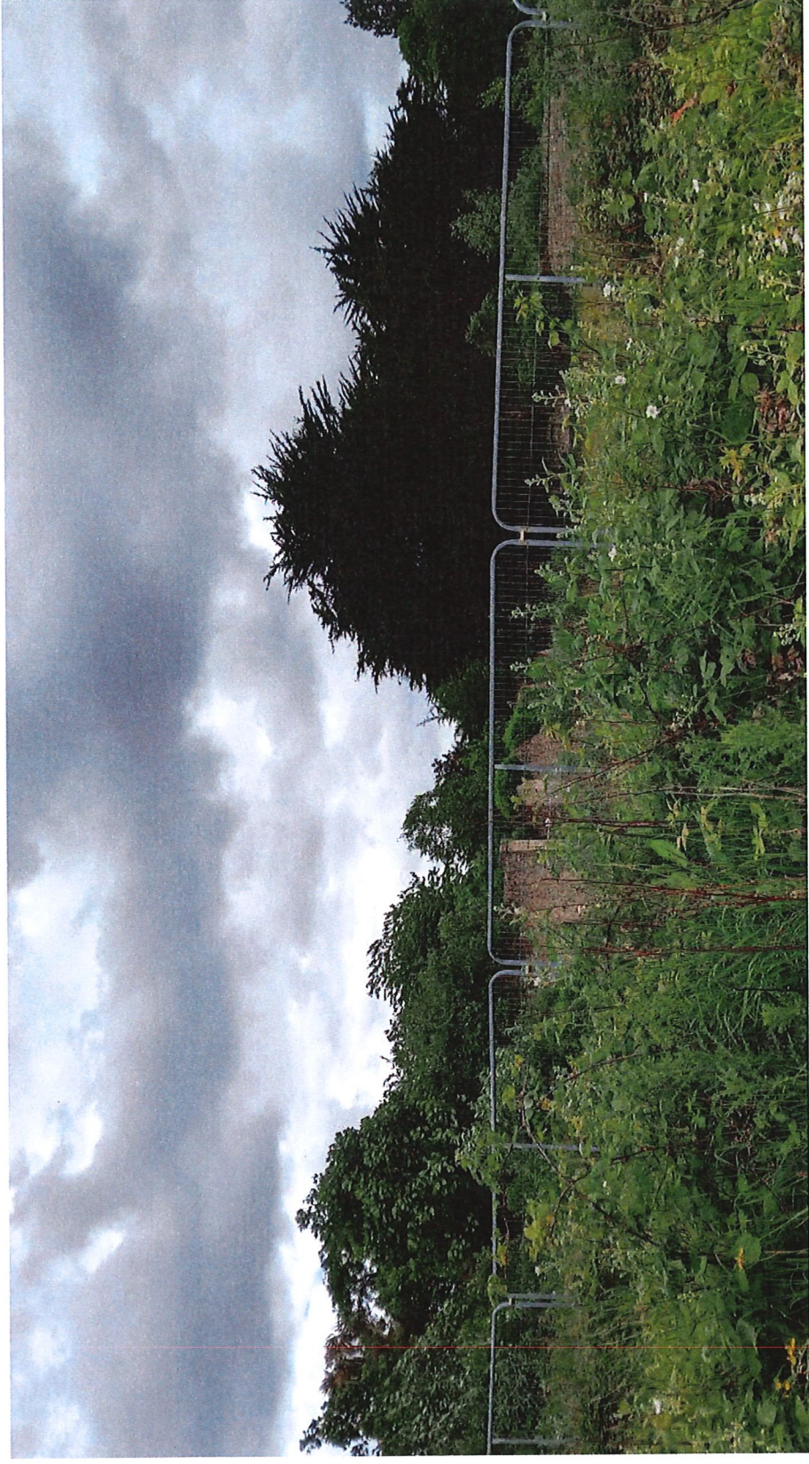
Fig. 13 — View southwest - 1837-1865 stone boundary wall between the rear 'The Garth', 'Thendara' and Hollywood House
